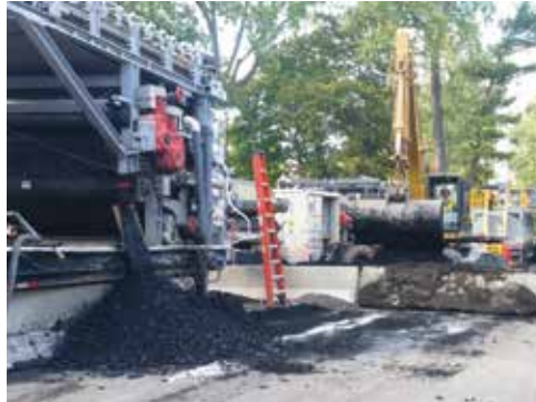
NEORS Green Lake Dredging, Shaker Hts., OH (Belt Filter Press)
